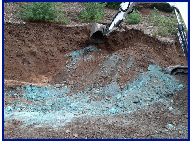
Copper flue dust reserves from the Bunker Hill Lead Smelter found near Kellogg. This is extremely high in lead, cadmium, arsenic, and mercury
